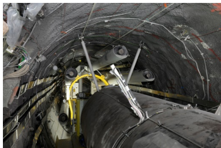
The emplacement drift is backfilled with granulated bentonite mixture using a specially developed machine. Source: © Comet Photoshopping, Dieter Enz
