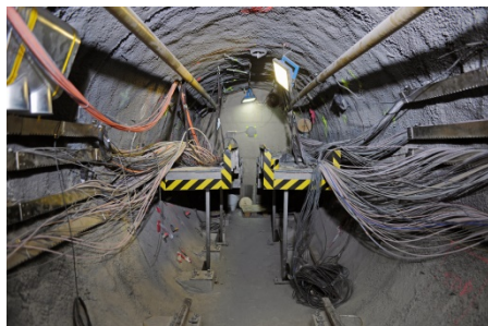
750 cables lead out of the drift and the surrounding Opalinus Clay and several thousand sensors continuously record measured values. Source: © Comet Photoshopping, Dieter Enz
