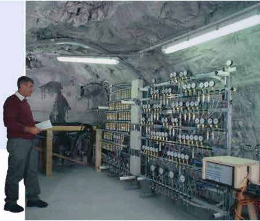
The Gas Migration Test (GMT) is being carried out at the Grimsel Test Site; lead organisation is the Radioactive Waste Management Funding and Research Center (RWMC) of Japan.
