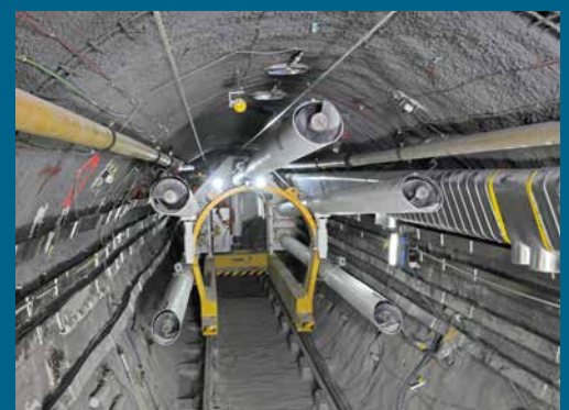
Setting up the FE demonstration experiment at the Mont Terri Rock Laboratory: Top: Bentonite blocks are used as pedestals for the test canisters. Bottom: The backfilling machine in the FE tunnel
